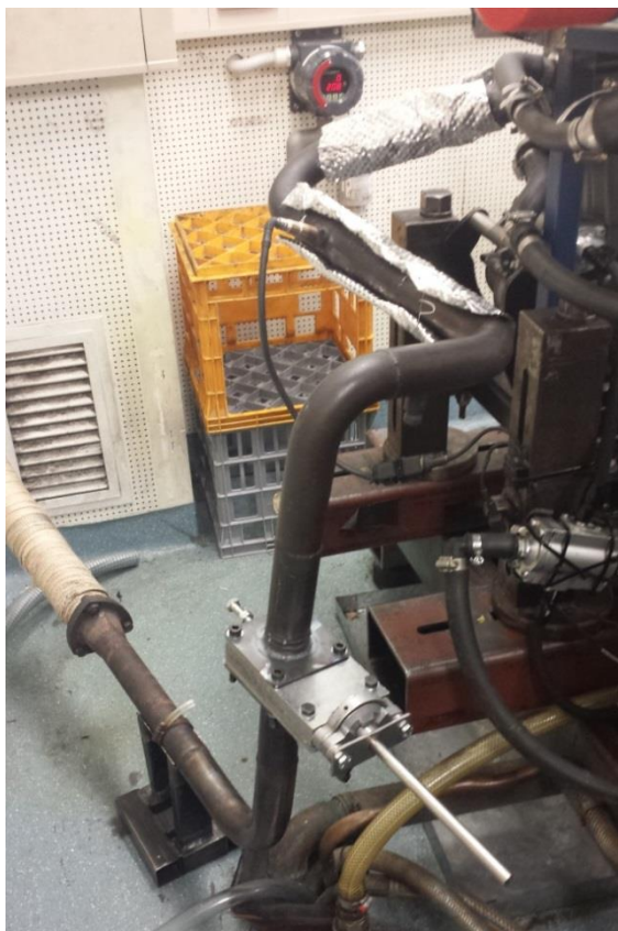
Figure 80: The dynamometer's exhaust system, including new brake.
