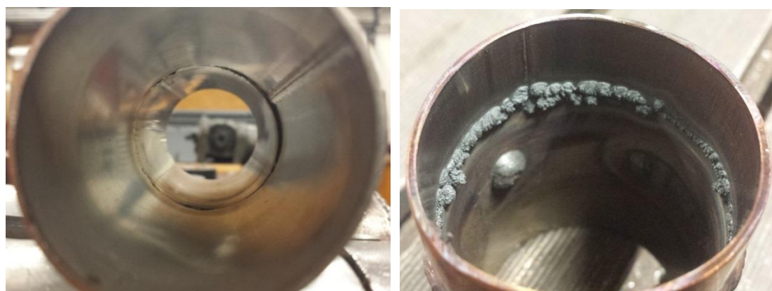
Figure 34: Left: Purged tube weld. The dark crescent is due to misalignment of the two tubes. Right: Unpurged tube weld. Note extensive crystallisation typical of unpurged exhaust welds in MMS's past.
